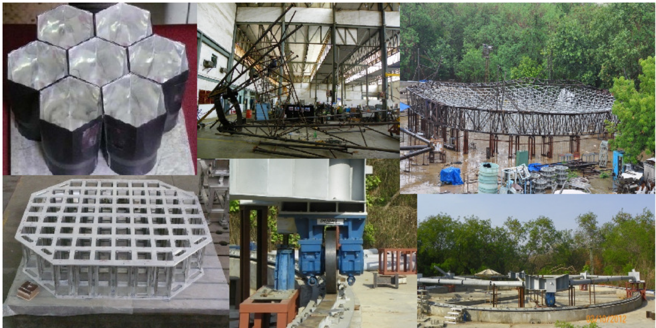
Fig. 4. Views of the ongoing installation of MACE near Hyderabad, Andhra Pradesh, South India.
